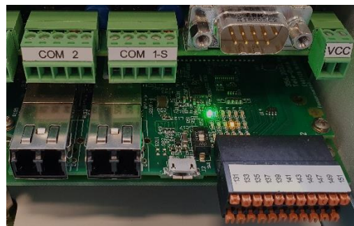
Fibre optical connection (2 x Ethernet-LC) at Level II; REG-DA Com ports at Level III
